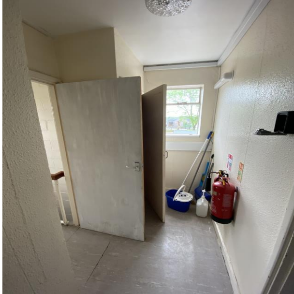
Photo number 1 – Door at head of stairs and electrical cupboard door. Replacement required.
